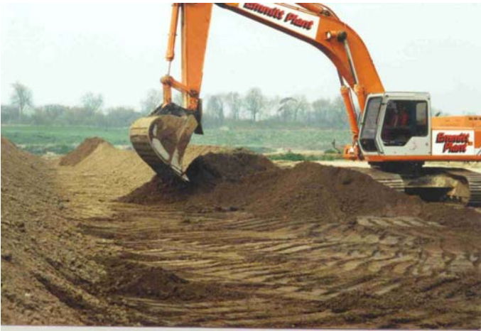
Example of the type of excavator and bucket used to place the Landscape20
